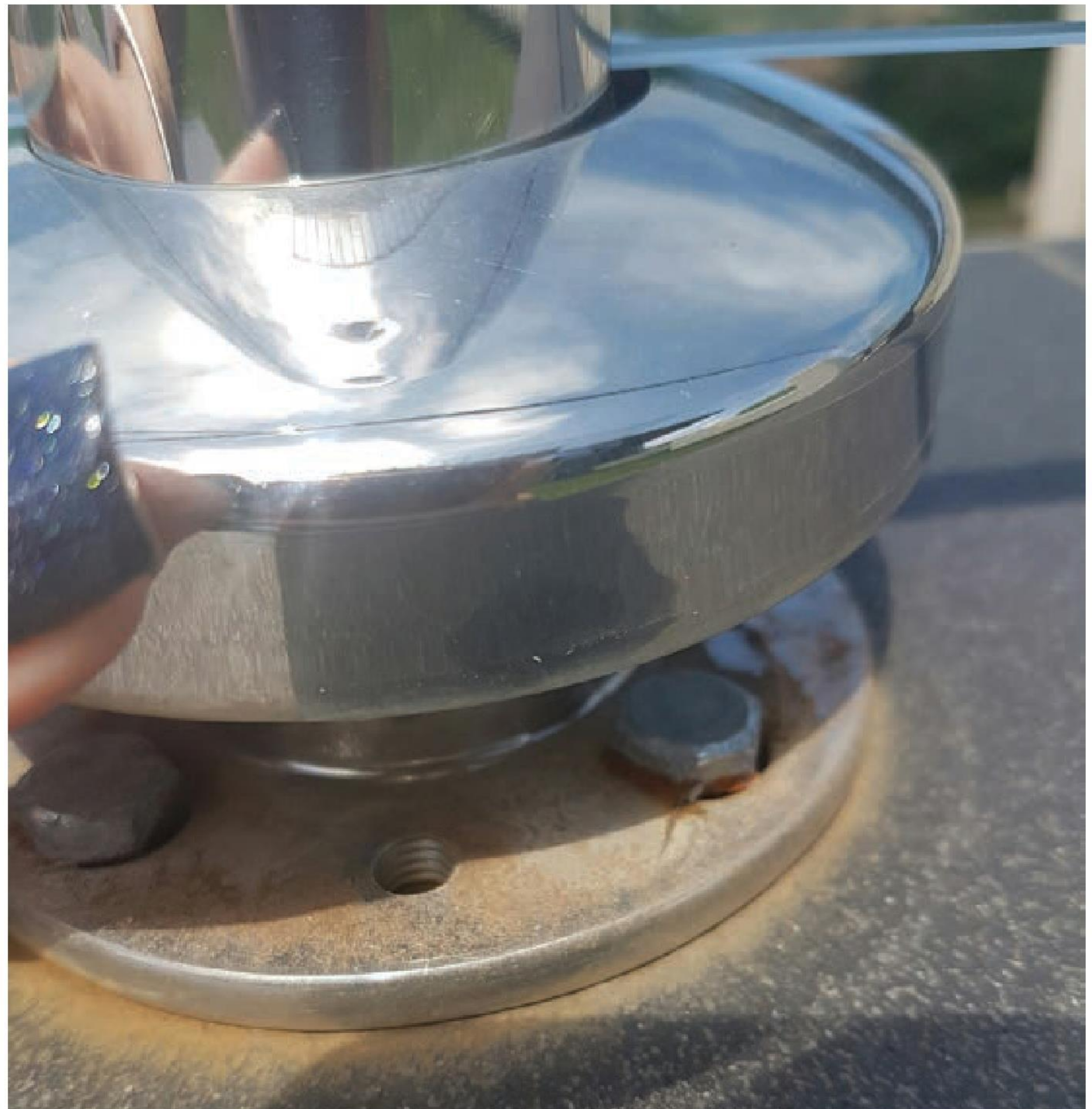
■ STL: Example of sub-standard stainless steel balustrade installation in KwaZulu-Natal.
