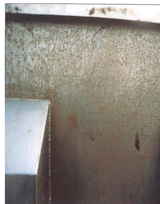
Mild steel contamination on 3CR12
