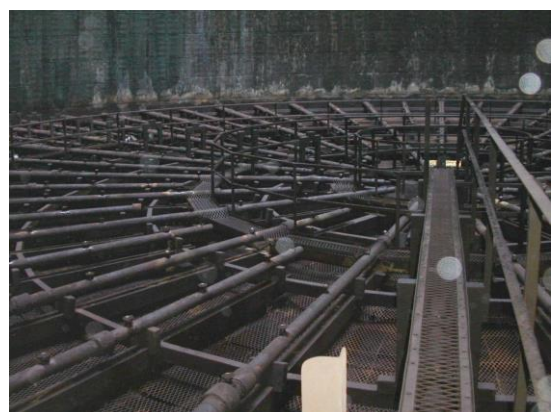
View of the X-GRID layers inside the cooling tower after 20 years' service. Diameter is approx. 52 metres. Picture courtesy of SASSDA.
