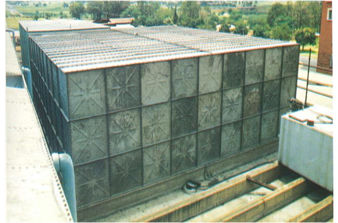
Boiler feed water storage tank installed at Rooiwal Power Station
