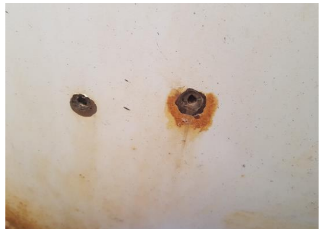
Microbial induced corrosion on the internal surface of a water tanker lead to concentration of deleterious chlorides causing pitting corrosion due to poor water chemistry
