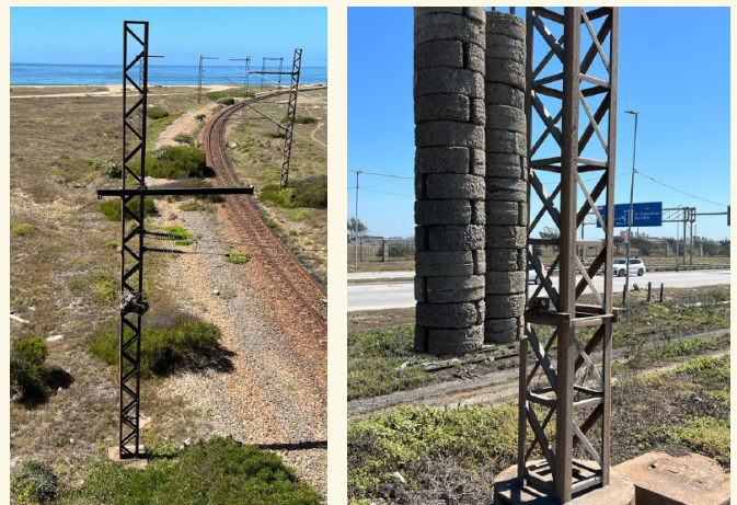
Figure 5: Pictures taken in 2022 illustrate the condition of the pylons over 40 years in operation.
