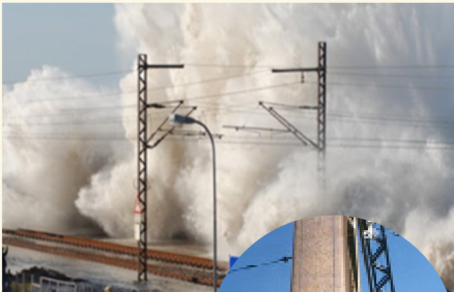
Figure 3 (a-b): 30 year inspection – taking note of the sea spray on the structures. Note: The original forming marks can still be seen on the metal surface, signifying the negligible metal loss.
