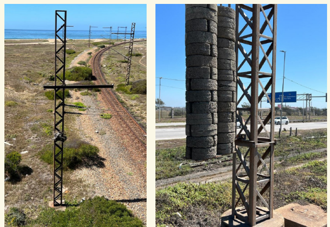
Figure 5: Pictures taken in 2022 illustrate the condition of the pylons over 40 years in operation.
