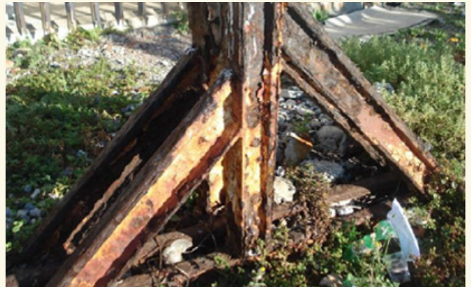
Figure 4: A carbon steel rail buffer in the same area showing excessive corrosion and subsequent loss of structural integrity.
